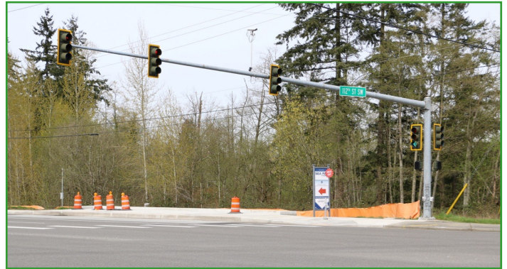
Southbound Airport Rd. at 112 th St. awaits electrical work, the last step before structure framing begins.
